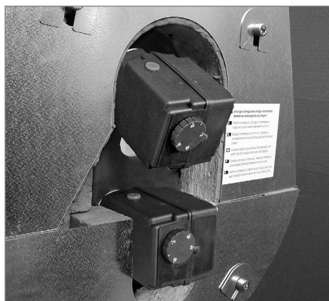
Installed electrical heating elements and flange insulation
