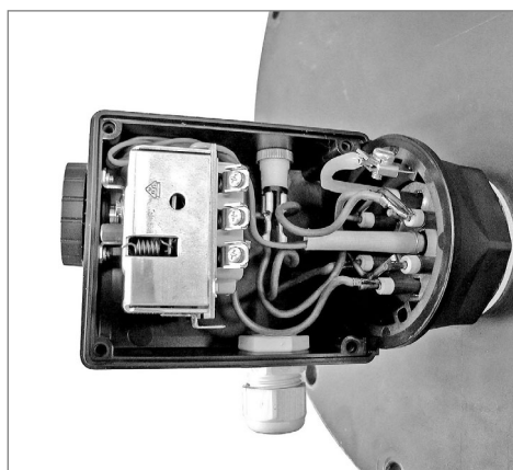
Connecting power cable
