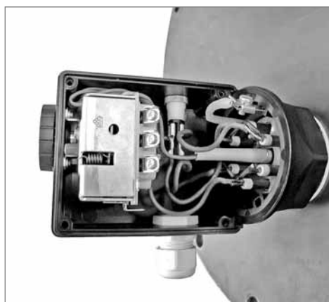
Connecting power cable
