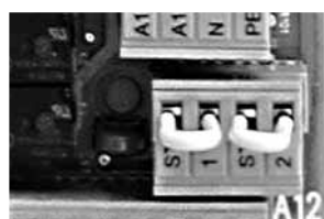
ST1/ST2 com 2 shunts
