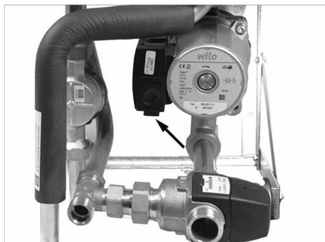
Fig. 3: Connecting the hot water pump
