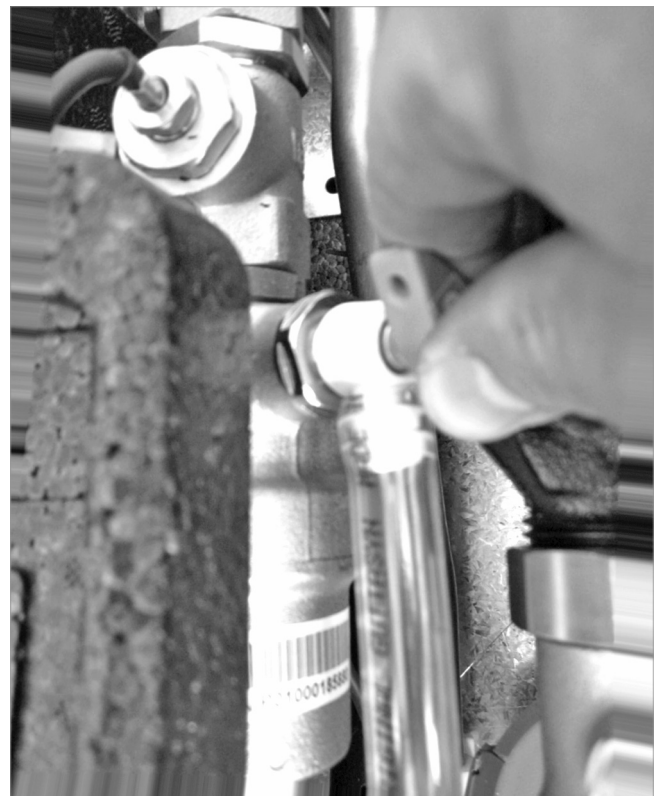
Fig. 11: Bleeding the deaerator
