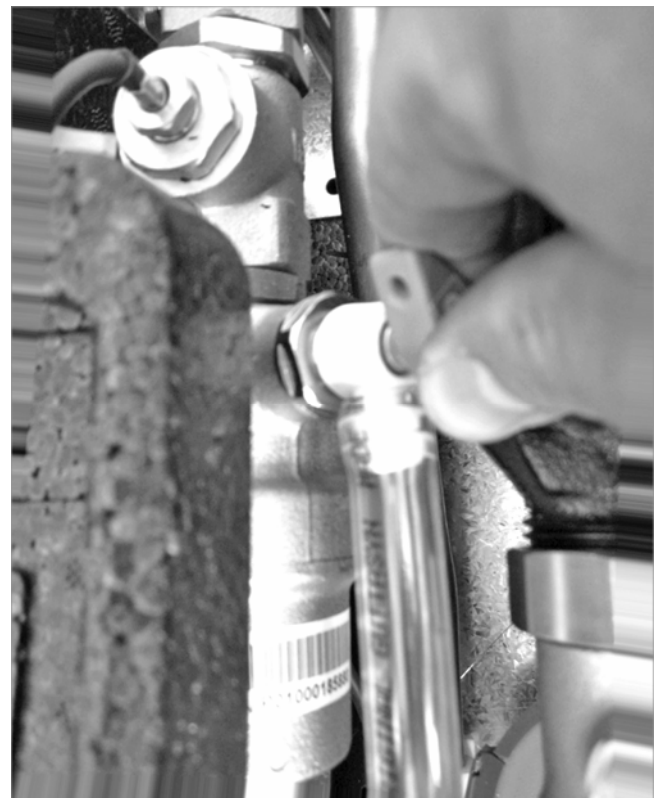
Fig. 11: Bleeding the deaerator
