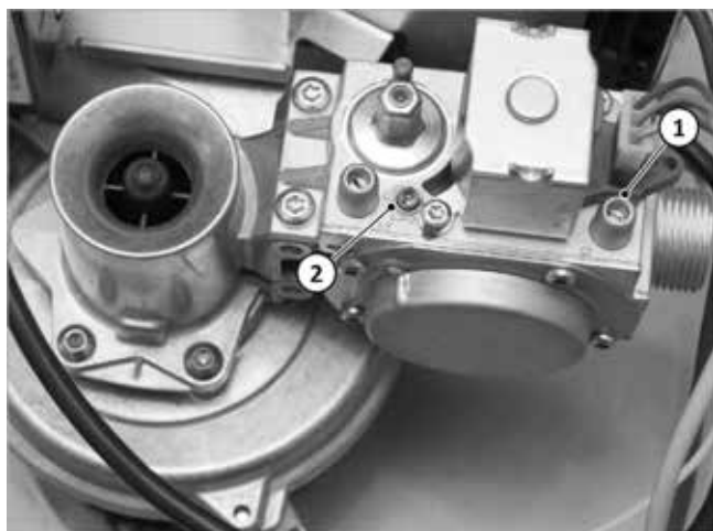
Fig. 30: Setting the burner
