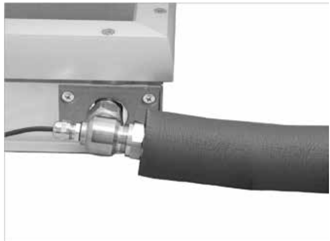
Fig. 72: Collector sensor on the solar flow, SolvisFera Diagonal
