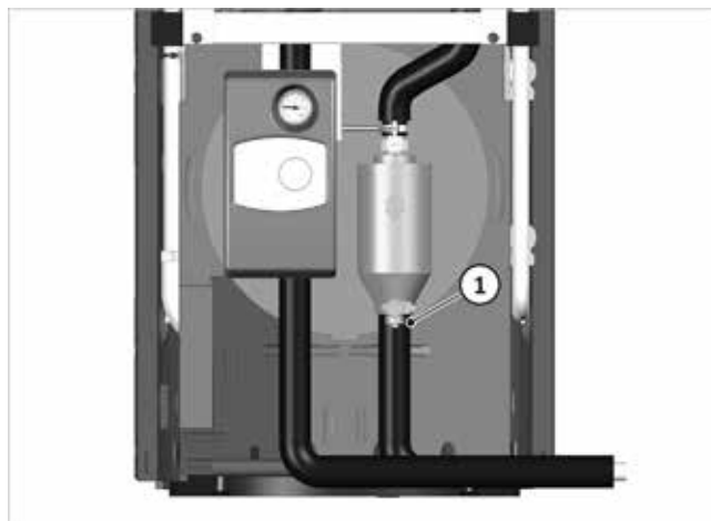
Fig. 82: Cleaning the sludge separator using the drain valve
