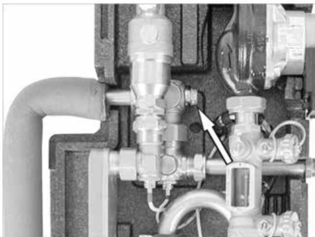
Fig. 17: Secondary-side manual bleeder
