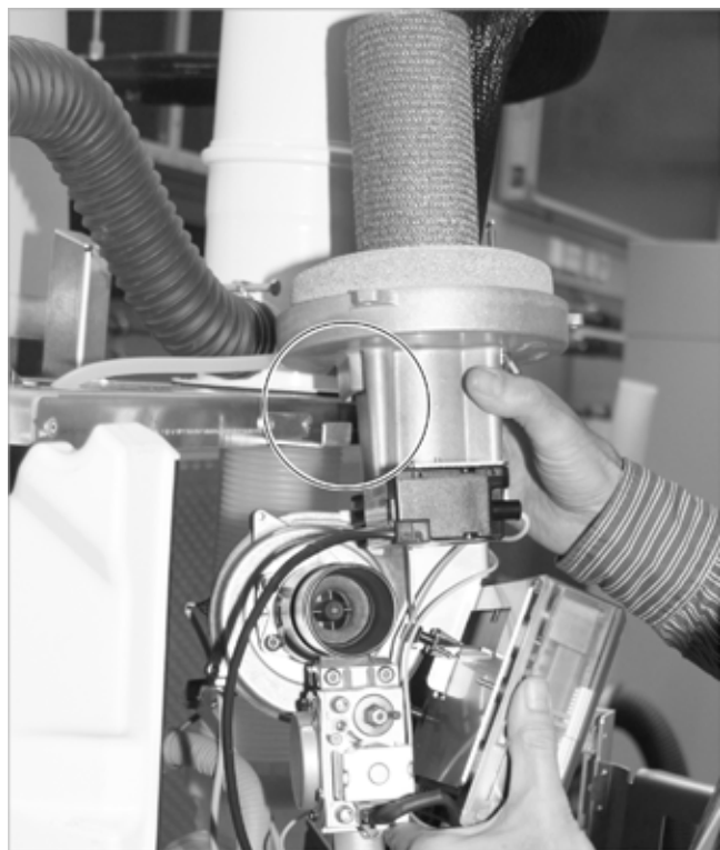
Fig. 112: Burner in maintenance position on the console
