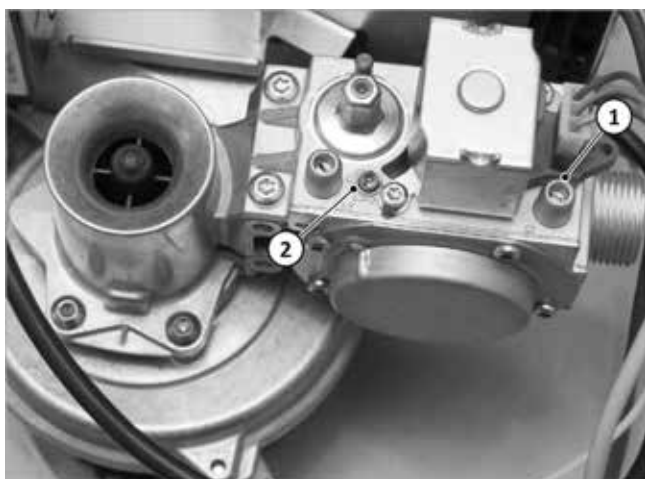
Fig. 113: Setting the burner
